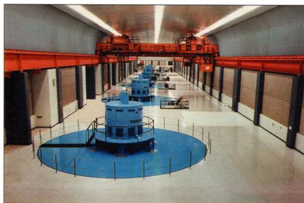
Hyatt Powerplant's six generators are capable of producing enough electricity to light the cities of Sacramento and Oakland.
