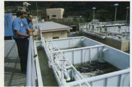
De aguas Recuperación Municipal—South Coast Water District, Orange Co., CA
