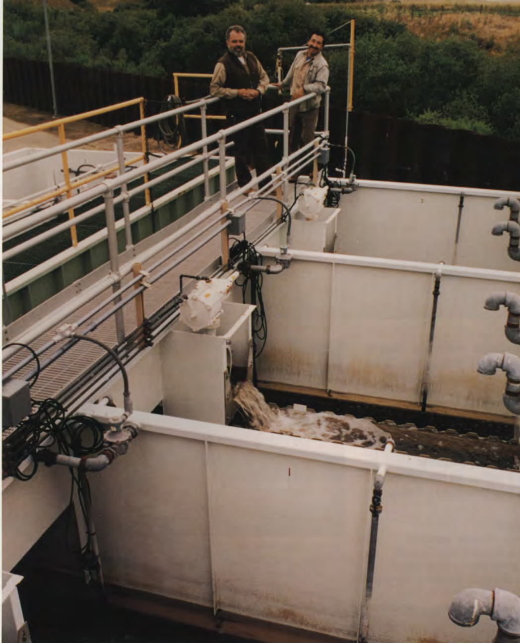
Lee Bickford and Mike Valverde view the Hydro-Clear® filter cells.
