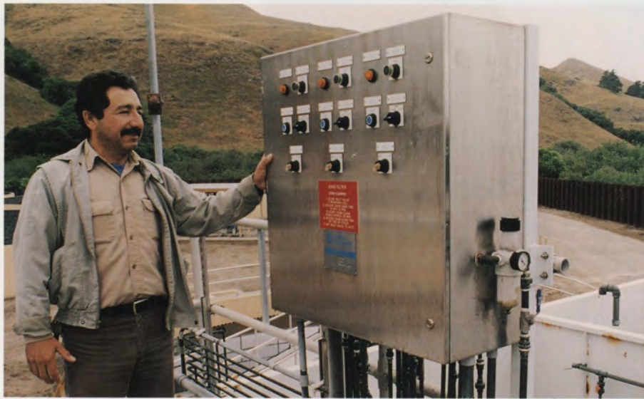
Mike Valverde at the filter control panel.
