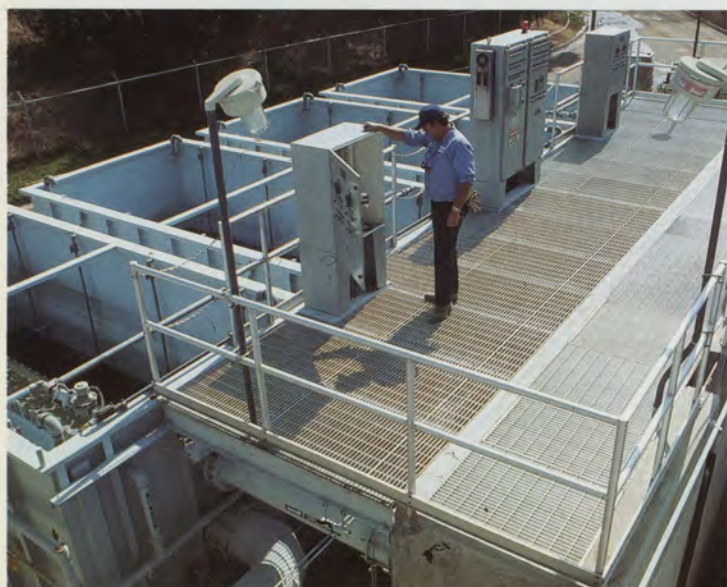
From top: filtered effluent approved for all reuses except potable. Silverthorn Nursery grows prize cactus plants with recycled water. Hydro-Clear® filter at Fallbrook.
