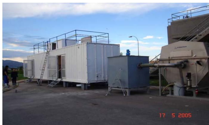
Figure 1. Overall view of the ACTIDisk ® demonstration plant at Castellón WWTP.
